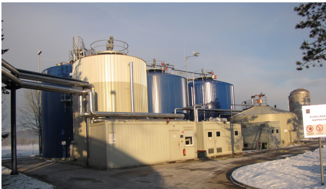
Figure 12: Biogas plant in year 2010. /17/
