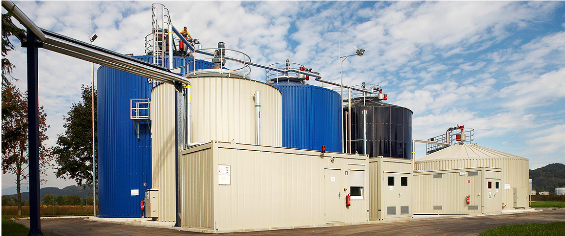
Figure 9: Biogas plant with reactors (from left to the right): front hydrolysis tank, back digester 1, digester 2, digester 3, and front anaerobic filter. /3/
