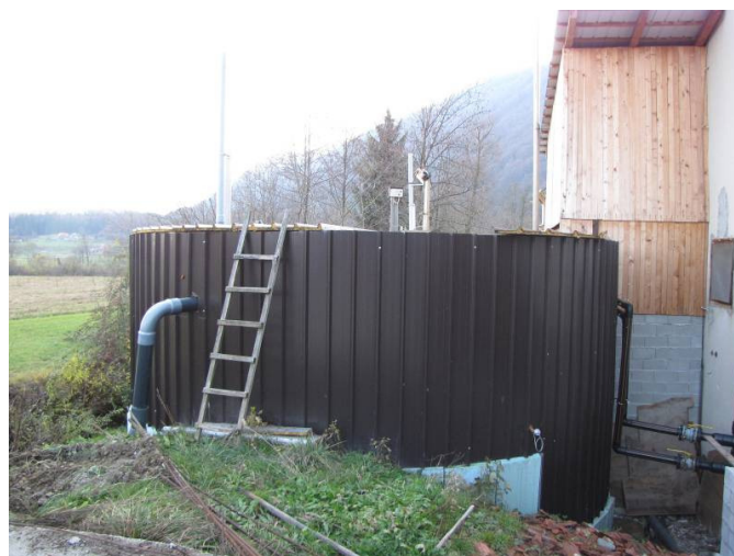
Figure 14: One of the digesters on biogas plant. /2/
